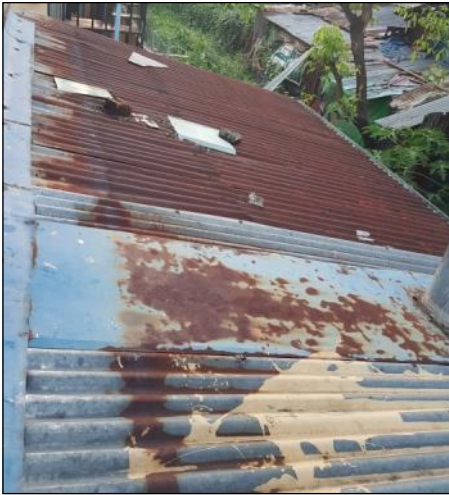
The old roof was in bad shape.
