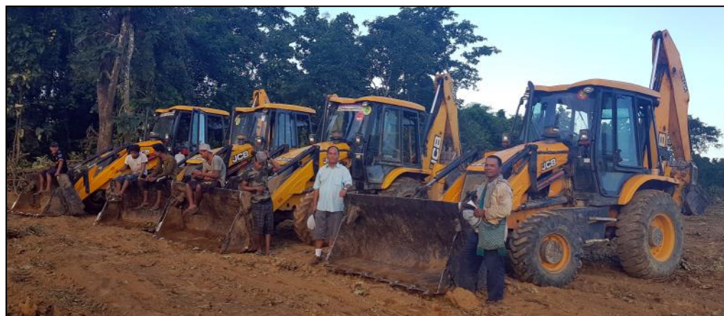
Palal with the four rented backhoes and drivers to clear the land
