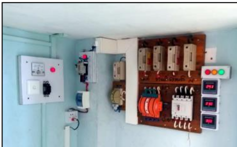
New electrical panel
