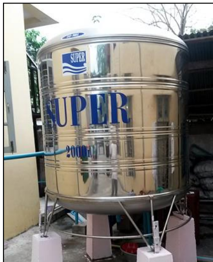
New 2,000 liter water tank
