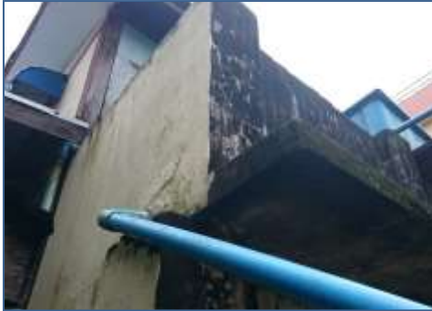
Leaky old water tank
