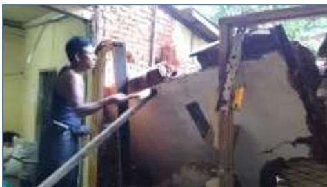
Back wall collapsed
